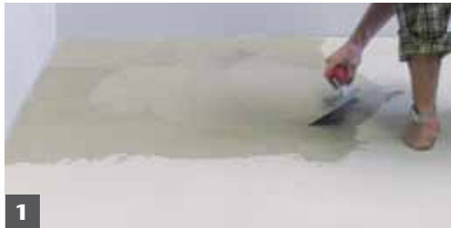
1 Apply loosely mixed modified thinset mortar to the substrate using a 5/16" V-notched trowel.
